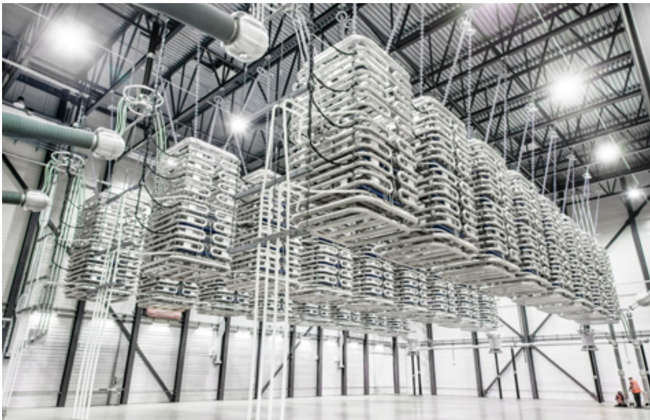
FIGURE 6. HVDC Light Valve Hall
