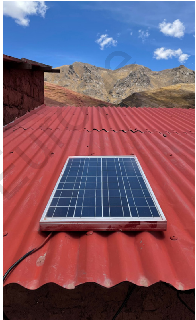
Solar panel installed in red roof on a house in the mountains of Peru. © Flavio Ferraz F
