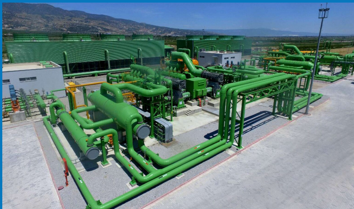
Greeneco Energy geothermal power plant in Sarayköy (source: EXERGY)
